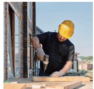
Outdoor work · Full of electricity, unlimited energy
